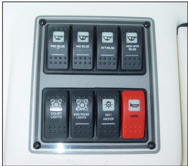
Port Helm Switch Panel
