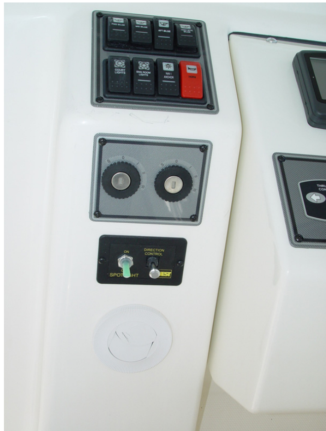
Typical Ignition Switches and Spot Light Control Panel
