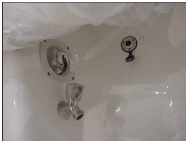
High Pressure Washdown Hose Connection
