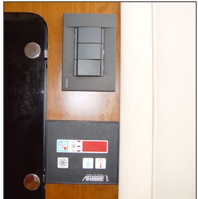
Cabin Overhead Light Switches and Air Conditioner Control Panel
