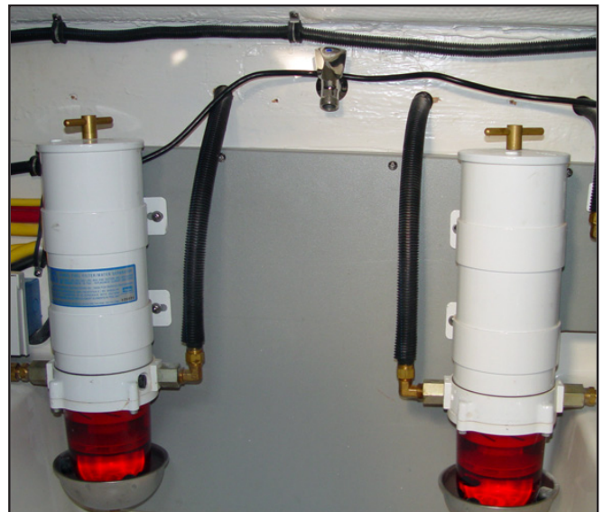
Fresh Water Washdown Faucet in Engine Room
