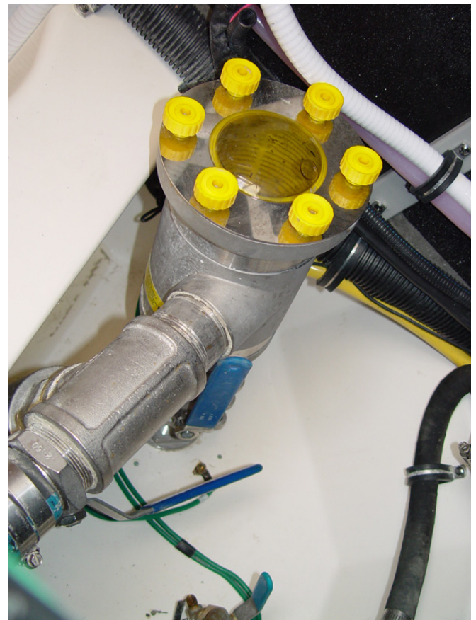
Starboard Engine Sea Strainer and Emergency Pump Out Valve
