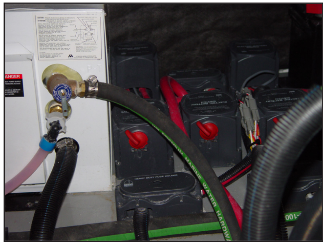
Battery Switches and Main Fuses
