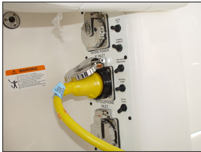
Shore Power and TV/Phone Inlet Plugs
