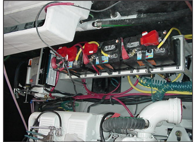
12-Volt Battery Banks
