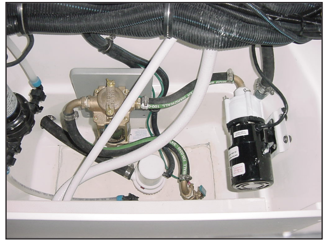
Air Conditioner Seawater Pump, Thru-Hull Valve and Strainer
