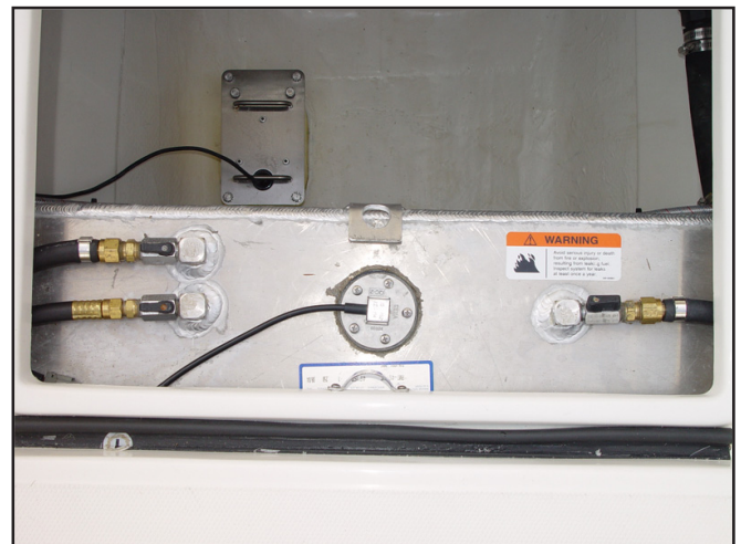
Fuel Supply Valves and Fuel Gauge Sender
